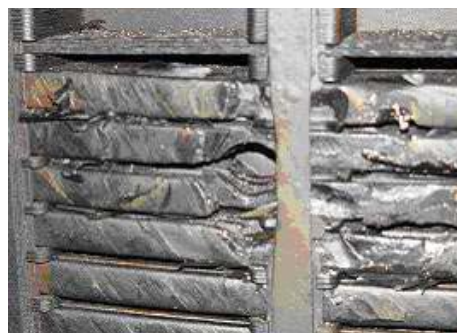
Figure 8 Failure of 330 kV winding contaminated with conductive oil by-products under lighting surge
