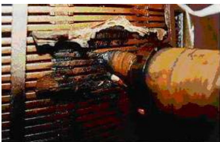
Figure 6 Short-circuit between coils due to introducing free water through poor bushing top sealing
