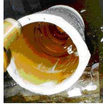
Figure 14 Internal staining with aged oil by-products containing metal colloids
